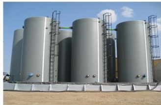
Tanks and pipes
